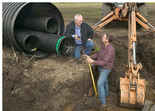
Soil scientist Norm Fausey (left) discusses site conditions and design features for a drainage water management and recycling structure with drainage contractor Paul Pullins.
